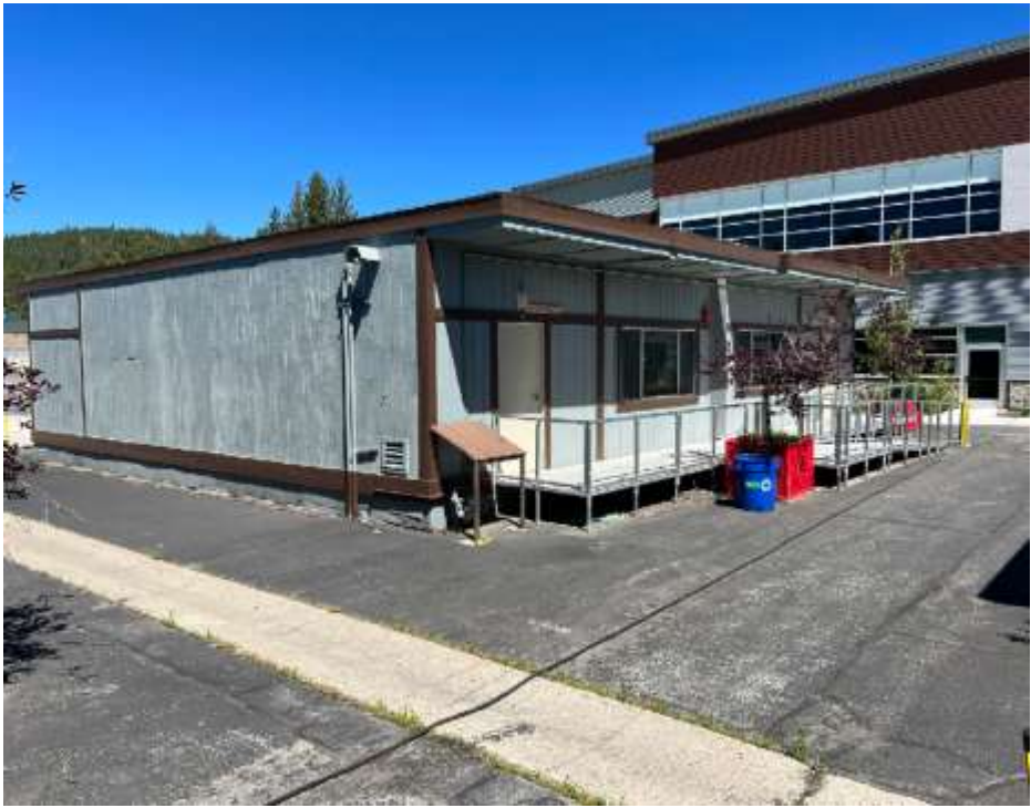
Cracked asphalt needs repavement
