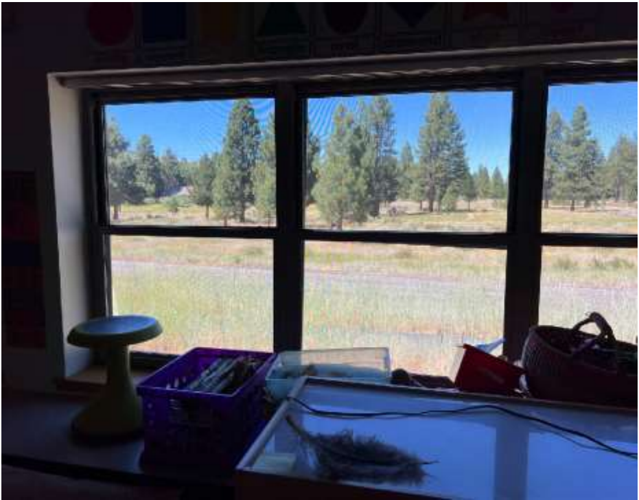
Snow removal access needed for windows
