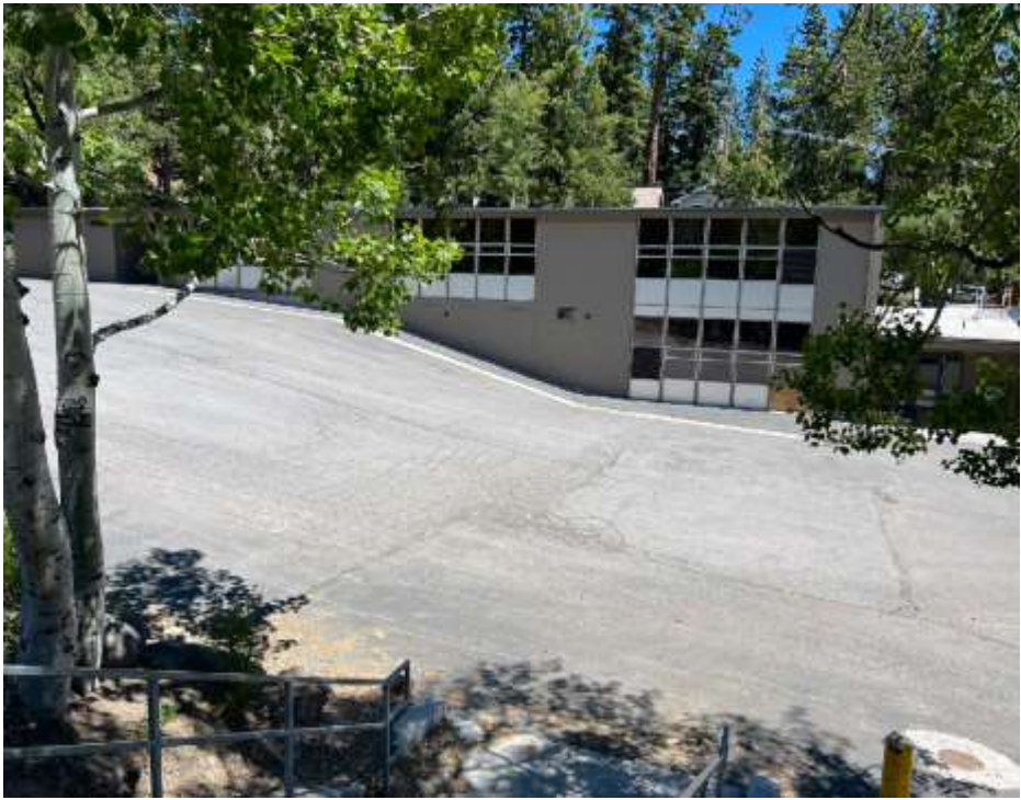
Paving upgrades needed
