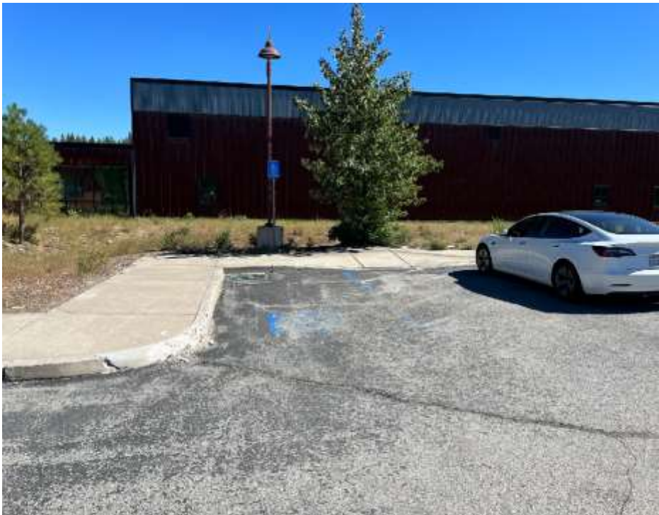
Asphalt needs resurfacing and restriping
