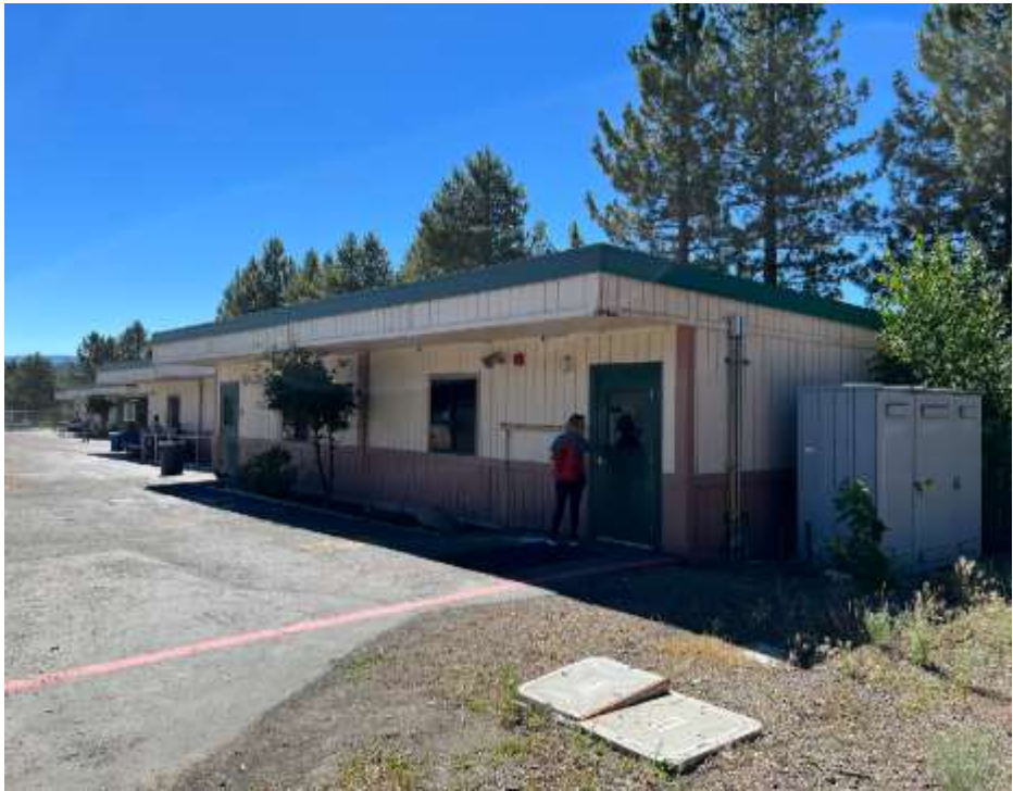
Portable roofing replacement needed
