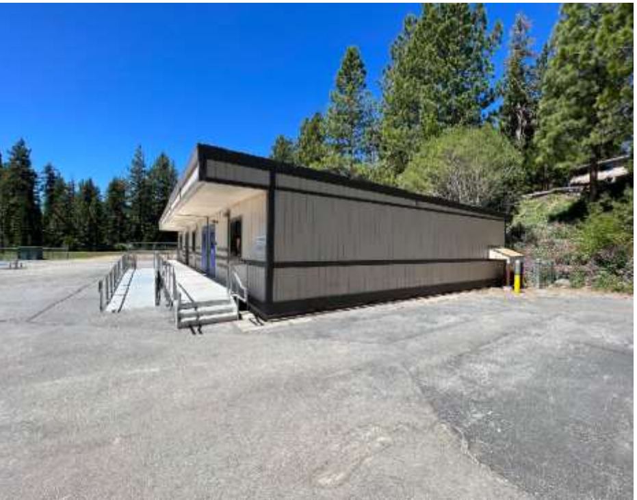
Portable roofing needs replacement
