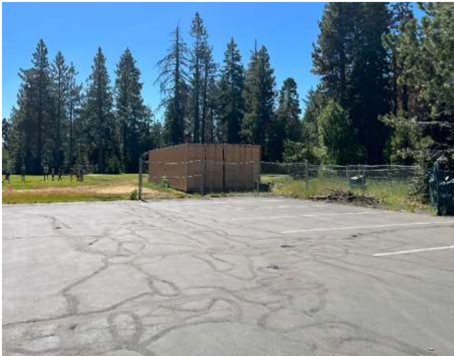
Cracked asphalt needs repaving
