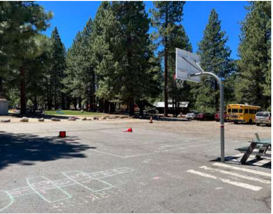
Hardscape needs upgrades
