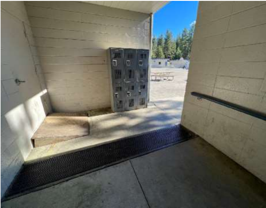
Required accessibility upgrades
