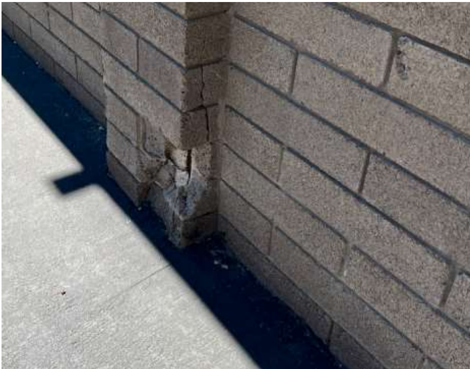
Ongoing deferred maintenance
