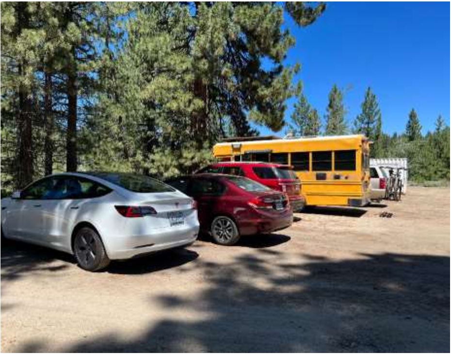
Parking lot needs paving and striping
