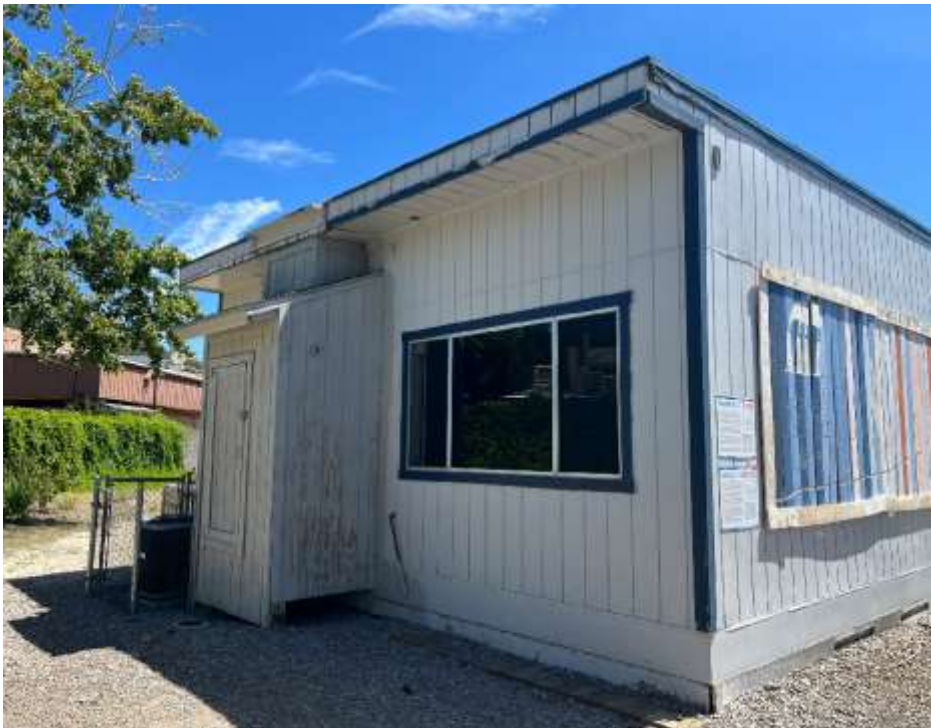
Exterior upgrades needed
