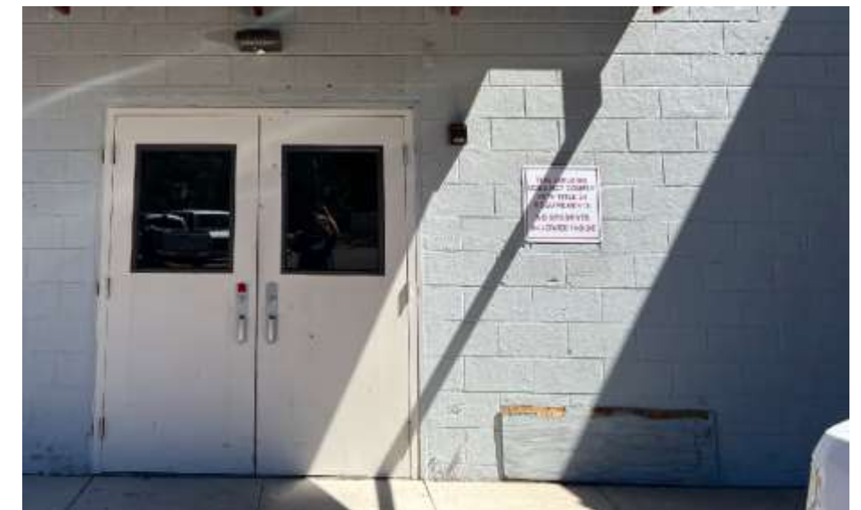
Some outdated buildings in need of replacement or modernization at high schools
