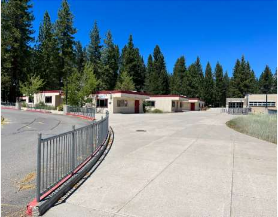
Concrete curb and sidewalk replacement needed
