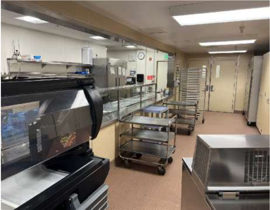
Kitchen upgrades needed
