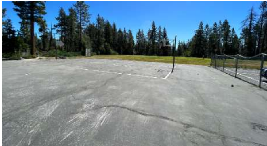
Repairs to paving from snow removal damage
