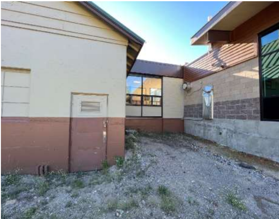
Upgrades needed for exterior windows, doors, and finishes need replacement
