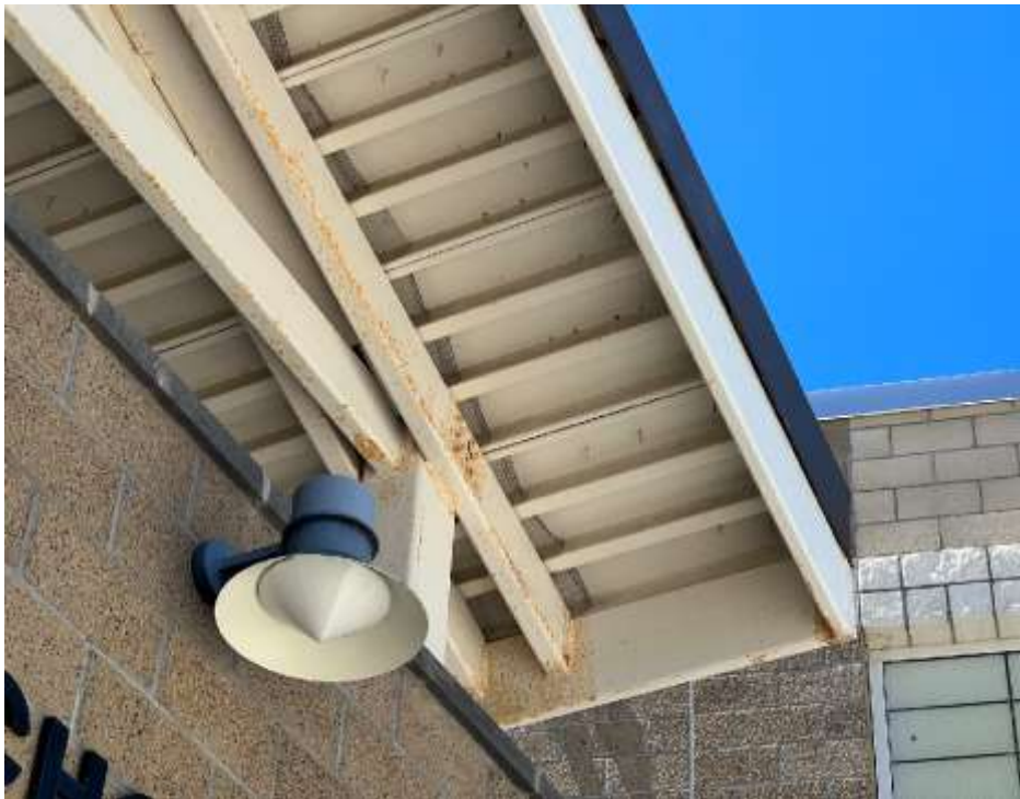
Rust at entry canopies
