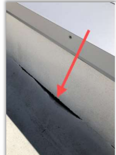
Membrane is cracked at the base flashing
