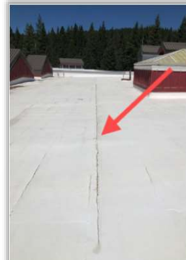
This crack is approx. 150 feet long
