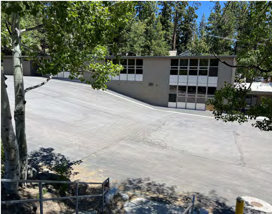
Paving upgrades needed
