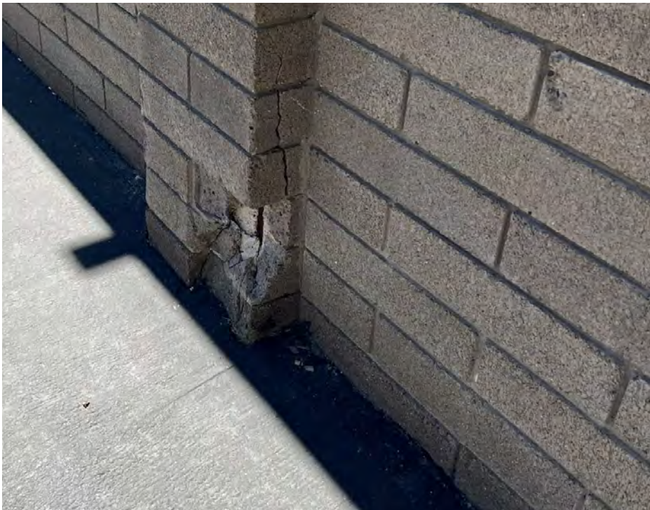
Ongoing deferred maintenance
