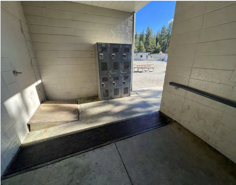
Required accessibility upgrades
