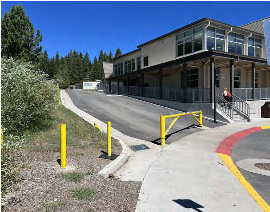
Single pane windows need replacing
