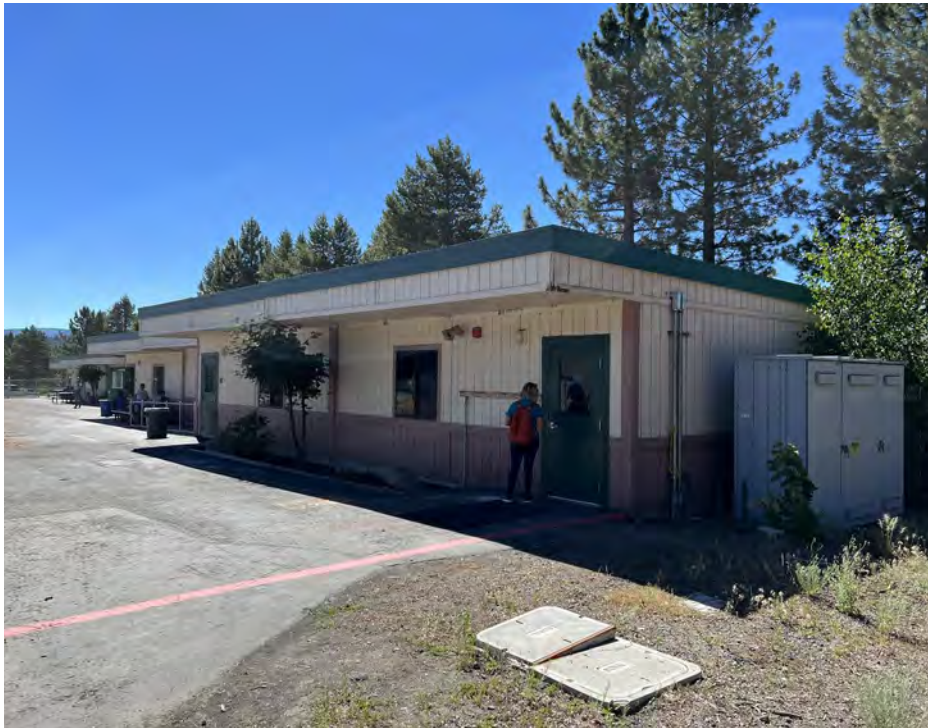
Portable roofing replacement needed
