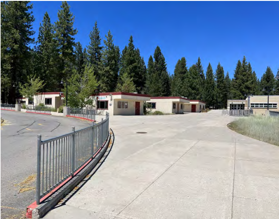
Concrete curb and sidewalk replacement needed
