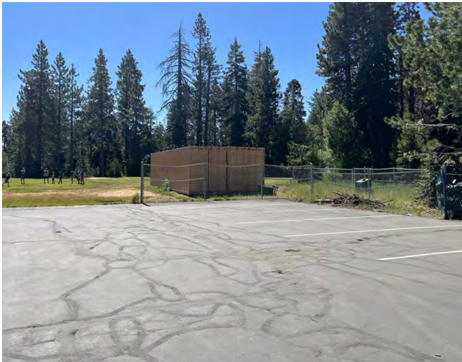
Cracked asphalt needs repaving
