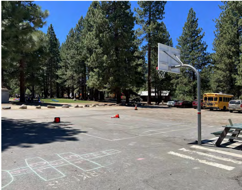
Hardscape needs upgrades
