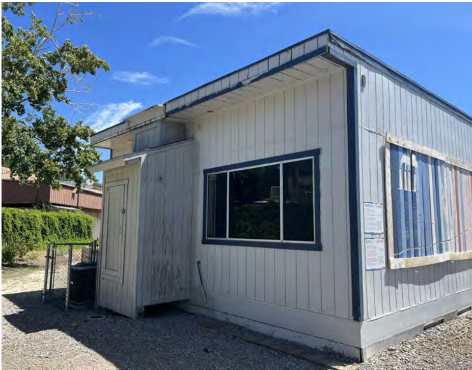
Exterior upgrades needed
