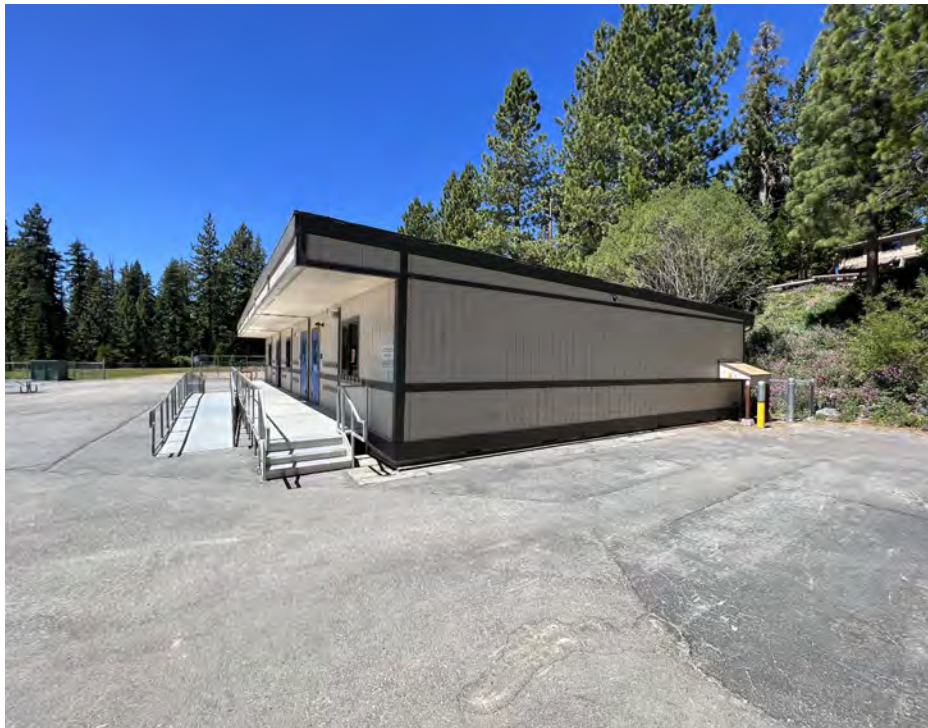
Portable roofing needs replacement
