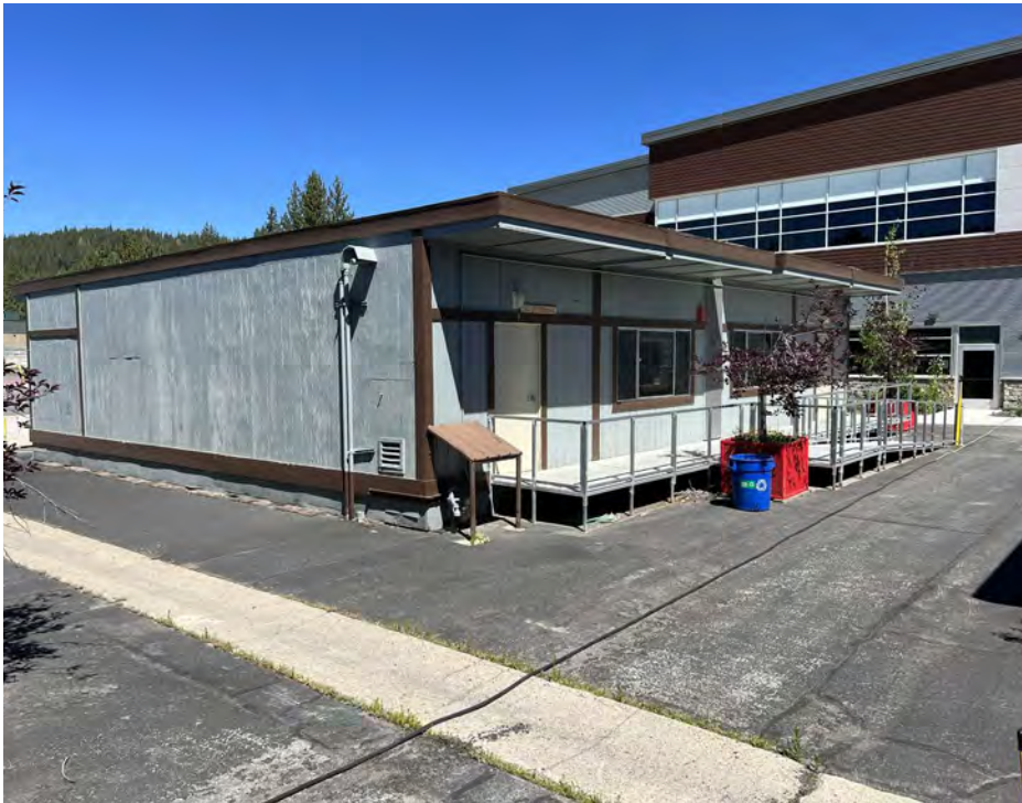
Cracked asphalt needs repavement
