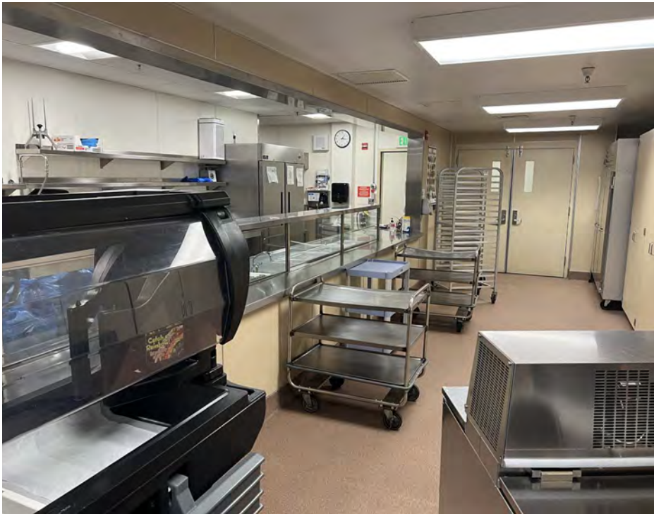
Kitchen upgrades needed
